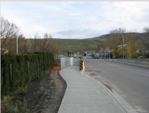
One costly project was the Fulton Bridge retrofit to add pedestrian access
